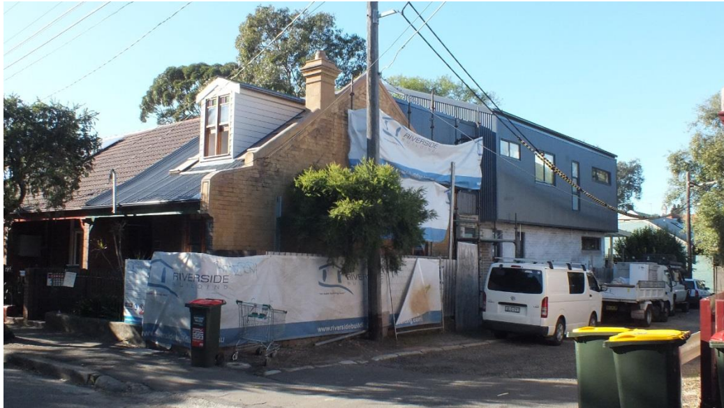
Figure 16 — Rear addition under construction to a single-storey Victorian residence on the corner of Camden and Princes Street in close proximity to the subject site (Source: NBRS+PARTNERS, May 2015)
